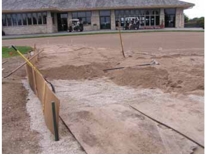
Once the layers of the existing green and the new expansion were matched, the boards were removed and used on the outer edge.
